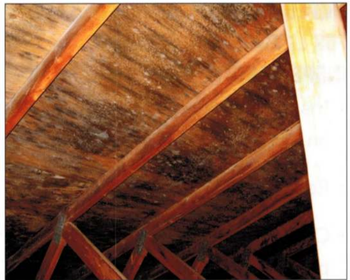
Inadequate ventilation in this attic space has resulted in decayed sheathing.
