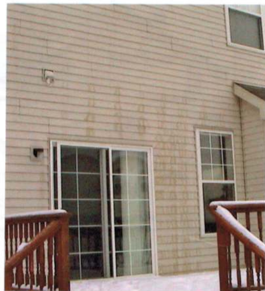
Staining on siding indicates severe condensation. Photo courtesy of Roger Hankey.
