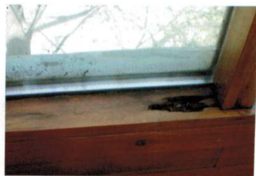
Water damage and rot on the interior sill of this window is a result of condensation, which commonly occurs with single-pane or poorly insulated glazing combined with high interior humidity levels.
