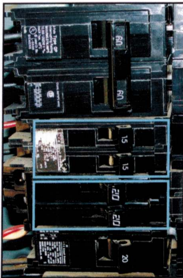
This photo shows the difference between two-pole tandem and single circuit breakers. The tandem circuit breakers are highlighted. From top to bottom, there is a 60-amp two-pole circuit breaker; a 15-amp tandem circuit breaker ( highlighted ); a 20-amp tandem circuit breaker ( highlighted ); and a 20-amp single-pole circuit breaker.
