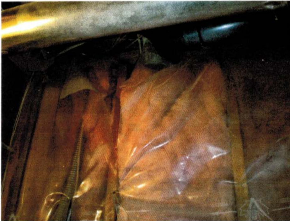
Damaged polyethylene film such as this is an ineffective vapor barrier, and an even more ineffective air barrier.
