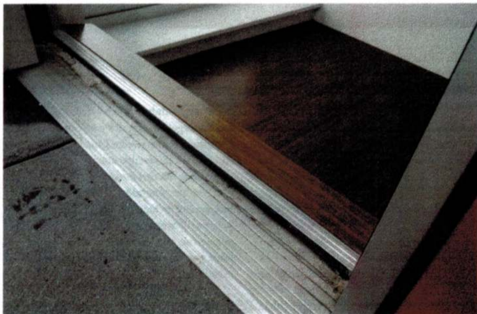
The photo above and the photo at the top of page 10 show a high-end out-swing commercial storefront door. This was very exposed but well-engineered. The sweep on this door locks into the threshold, and the hinges have a weather-proof cover.
