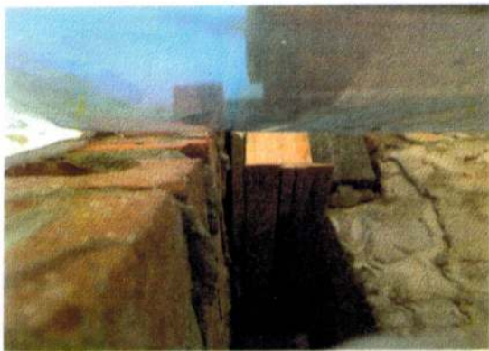
The brick veneer and sheetrock (left) and the chimney (on the right) has an embedded header between them. This picture—used for instructional purposes—shows a properly installed embedded header. While it may not be visible, it frequently lacks proper clearances.
