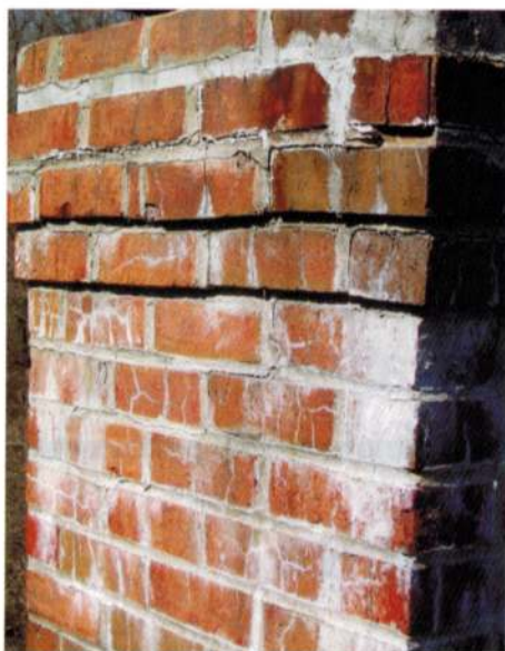
Here's an example of exterior colorization changes. This is efflorescence, which can be an indicator of moisture issues.
