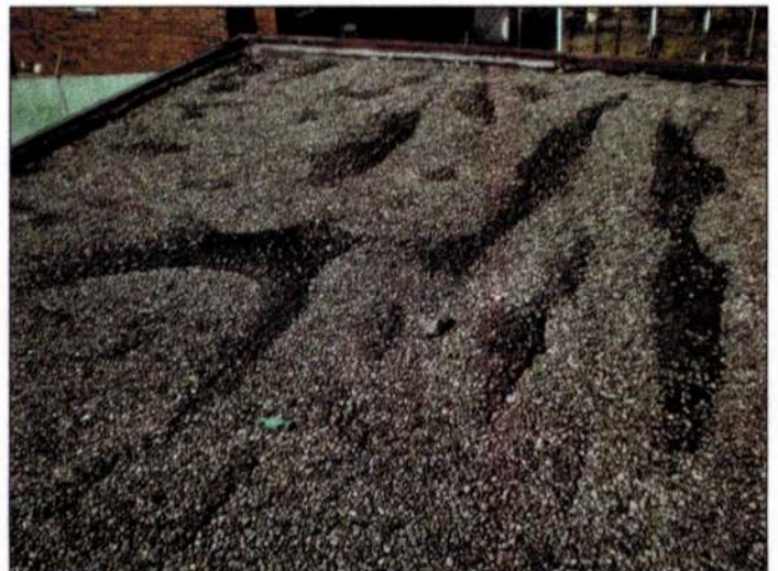
Blisters and loss of gravel on a built-up roof
