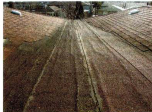
Membrane slippage and an open seam on a mod bit roof between two sloped roofs
