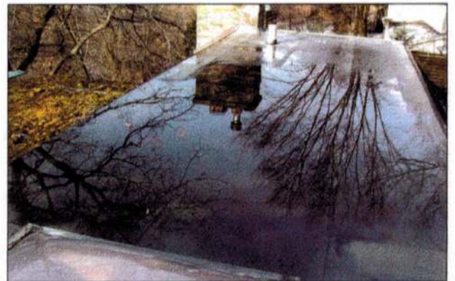
Water ponding is a common problem with flat roofs
