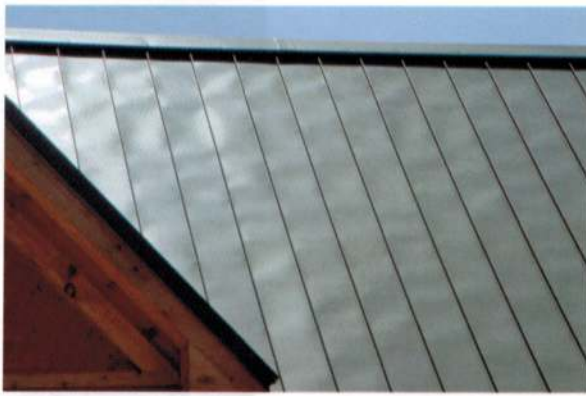
Oil canning on metal roof Photo courtesy of John Stortz & Son
