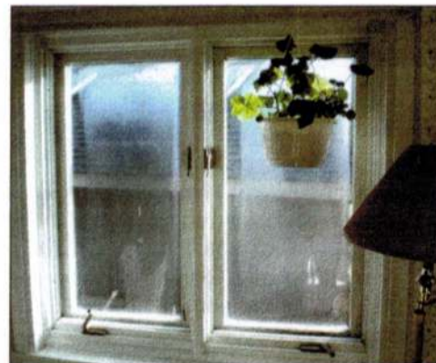
Lost seal resulting in condensation between the panes.
