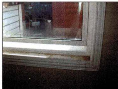
Excess condensation resulting in moisture accumulation at interior window sill and casing.
