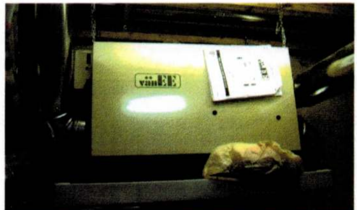
The cold-side ducts of this HRV unit leading to the exterior are not insulated.
