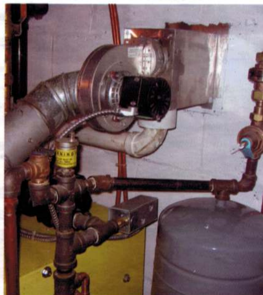
Direct-vent using galvanized steel.
