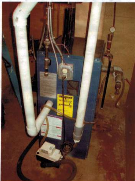
Direct-vent system using PVC pipe.
