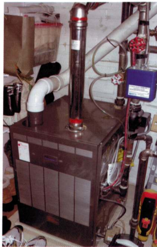
This boiler has a plastic intake and a steel exhaust—the condensate line on this one is not properly attached.
