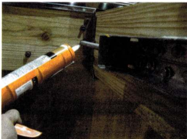
Figure 4. To keep out water and insects, the author caulks all holes drilled through the house. Note that he installs the brackets 6 to 8 inches away from ledgers, rims, and other framing members. The distance makes it easy to caulk holes in the rim joist, as well as access the brackets with a wrench or drill.
