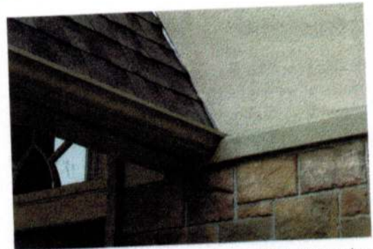
There is no kickout flashing on this new home. This is likely to be a problem area.
