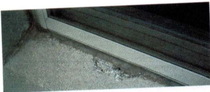
Workmanship is often an issue, as seen on this windowsill.
