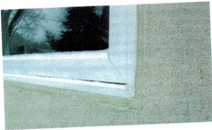
The joint between the synthetic stucco and windows is a vulnerable area. This system appears to be in good condition with a well-caulked joint.
