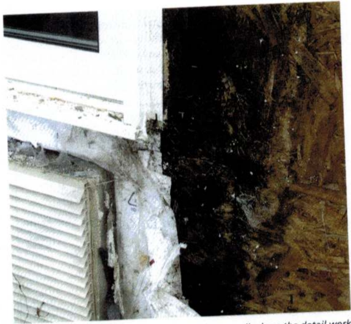
Here's what it looked like when we opened up a wall where the detail work was not so good.
