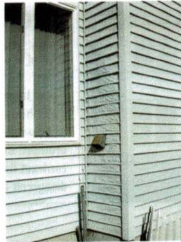
Vinyl siding damaged by reflected sun from nearby window.
