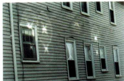
Buckled vinyl siding due to reflected sunlight from windows in adjacent building. Note the "stars" of reflected light. (Photo courtesy of Don Lovering)
