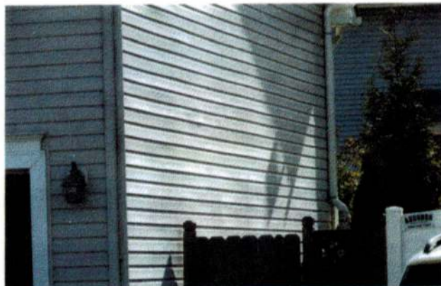
Siding is wavy because of poor installation.
