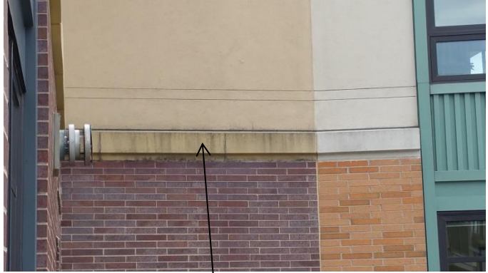
Exterior above window looks like this
