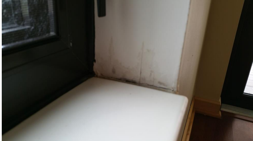
Water damaged living room wall & sill
