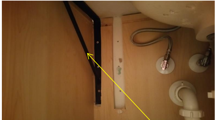
Support under sink
