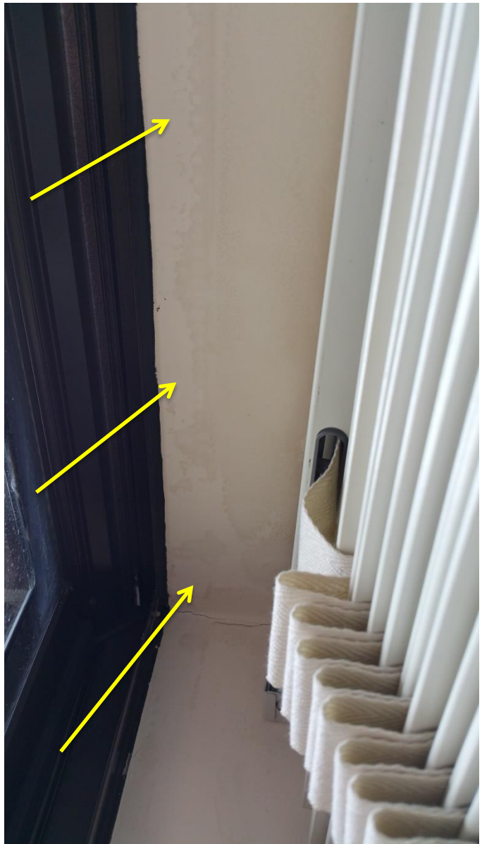
Water stained top of dining room window
