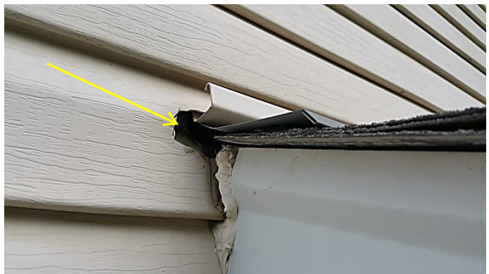
Hole in siding
