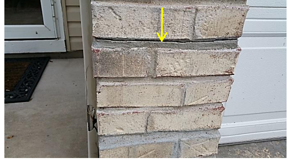
Loose brick veneer
